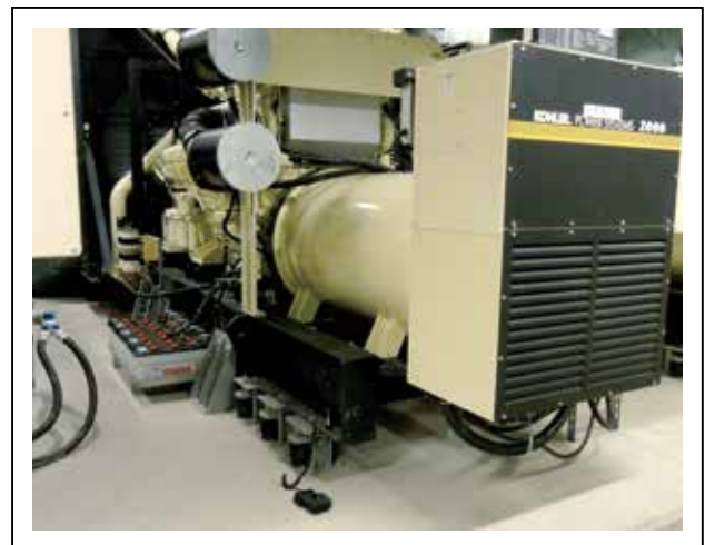
YS-EA used in Generators
