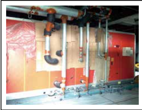
Air Handling+Piping System
